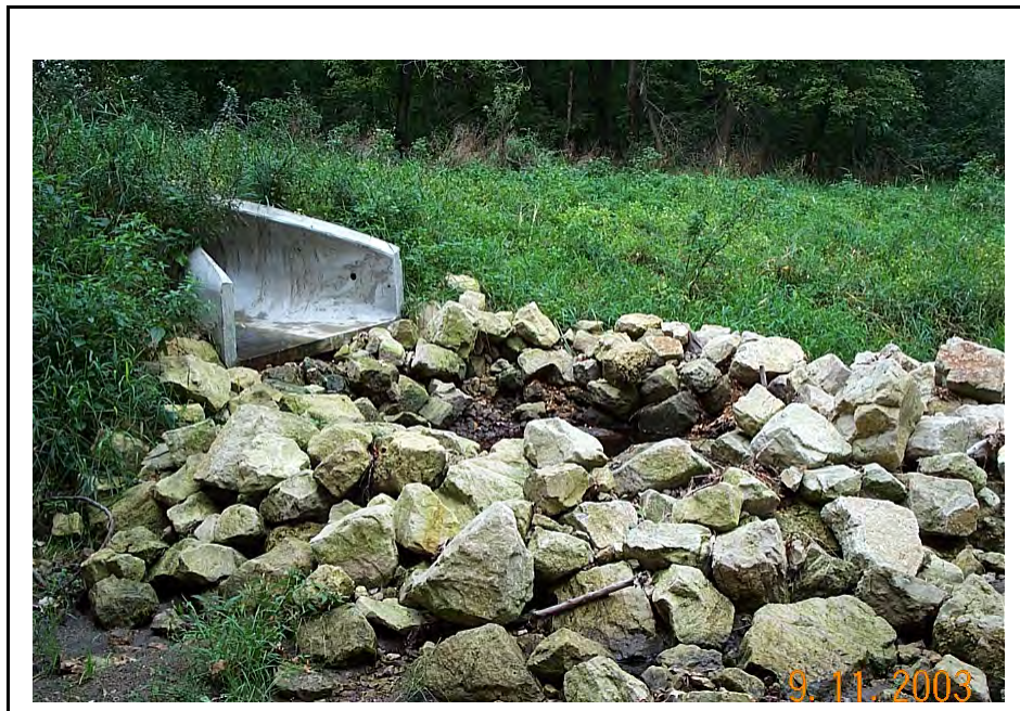
Figure 5-27 New Storm Sewer Inflow Upstream of Reach PC5A
