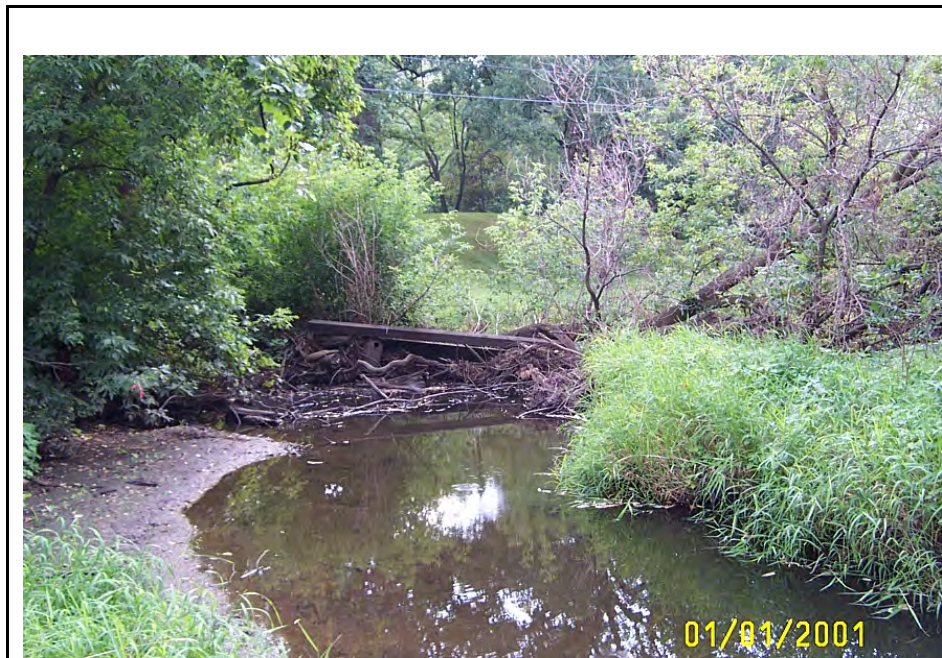
Figure 5-23 Reach PC2 Debris Jam
